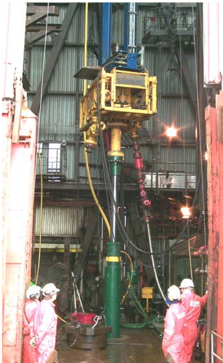
Fig. 10—The slip joint is pictured after installation below the surface flow tree on Transocean Searcher
